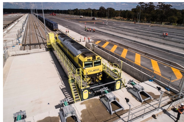
Locomotive traverser at Moorebank Logistics Park in south west Sydney, currently being completed xxxiv
